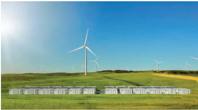
TESLA Powerpack UPS 100MW/129MWh, Jamestown, South Australia
